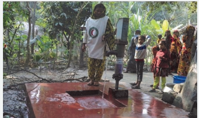
Figure: Rehabilitation of water point at Purbo Burir Char Community, Barguna Sadar
